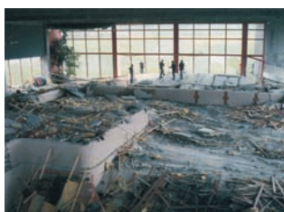
In 1985, the suspended concrete ceiling of an indoor swimming pool broke in Uster, Switzerland. The ceiling attachments of stainless steel exhibited no external defects whatsoever, but inside were completely destroyed in some cases due to stress corrosion cracking.
